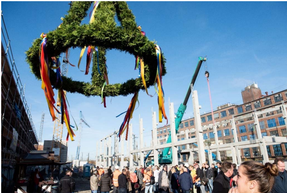
Photo 1: Topping-out ceremony at the new business premises at Gertrud-Knebusch-Strasse (© Zweckverband Abfallwirtschaft Region Hannover)
