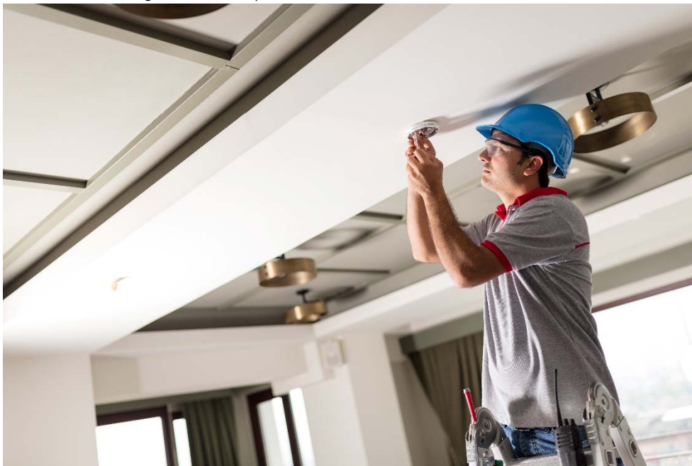
Photo 2: Among other things, fire detectors are installed throughout the building complex. (© iStock/nilimage)
